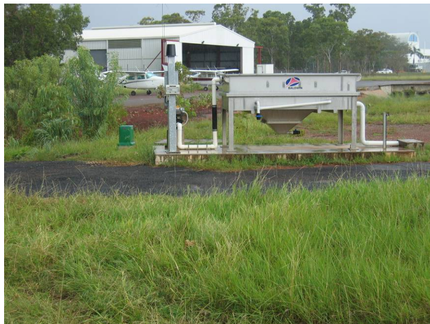
Figure 8: Example of plate-separator pollution control system installed by Darwin International Airport.
