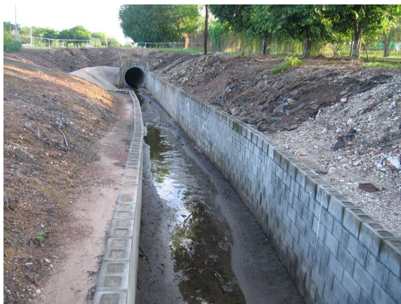
Figure 5: Example of a stormwater drain servicing the urban areas that flows into Rapid Creek.
